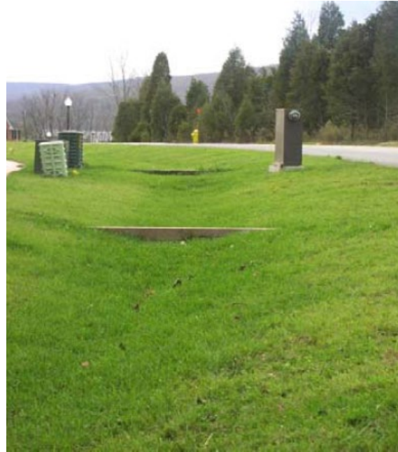
Figure 3-1: Example of Enhanced Grassed Swale (Figure 4.8.2 from TRCA & CVCs Low Impact Development SWM Planning and Design Guide)
