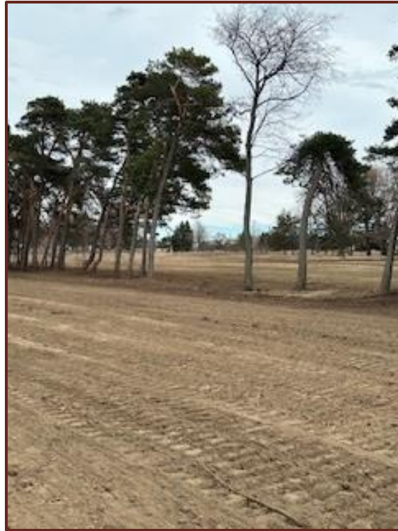
Photo 13. Removal of vegetation and grading carried out in the property (taken by others on February 16, 2024).
