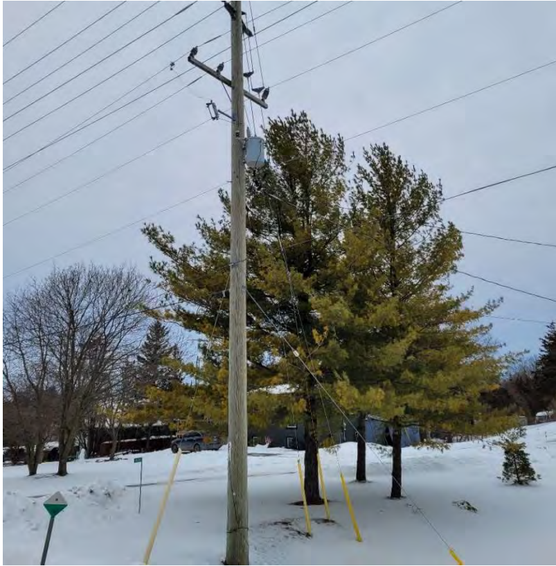
Photo 7: Hydro pole mounted transformer located along County Road 22 proximal to the Phase One Property
