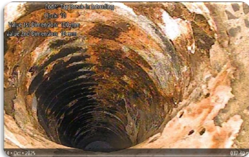
Severe corrosion of corrugated steel pipe compromising structural integrity
