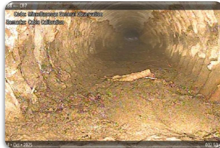
Severe corrosion of corrugated steel pipe compromising structural integrity
