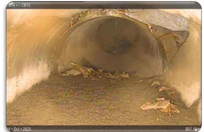
Cracked and missing section of concrete pipe with joint offset
